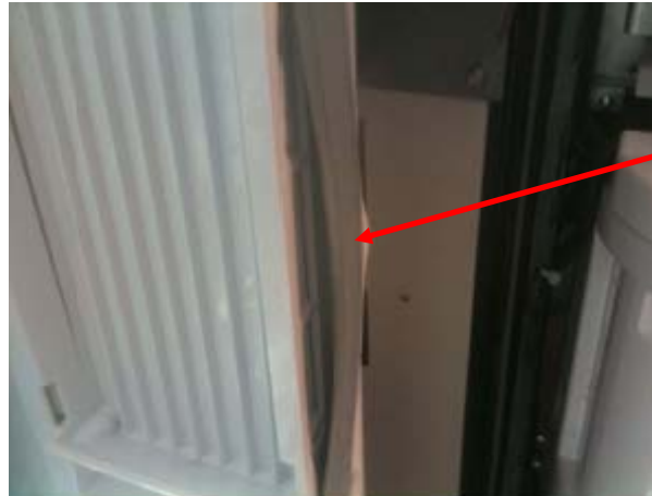
Metal bowed away from the Delivery Door area.
